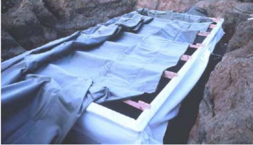
Fig.: The liner bag is first placed onto the centre of the auxiliary beams
